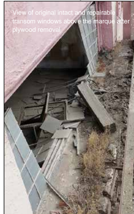
Original metal-framed transom windows with ribbed panes above the façade storefronts and doors after removal of plywood in August 2019.
